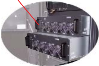
UPS POWER MODULES
